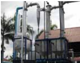
Water Scrubber and Chiller Scrubber
